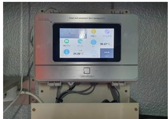
(c) Control panel
