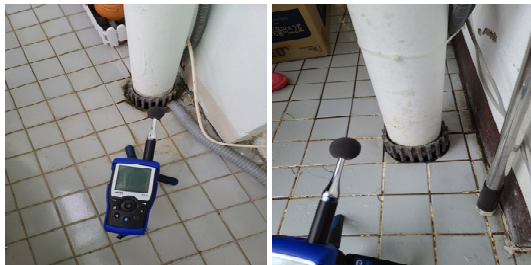
Fig. 4. (Color available online) Measurement site and details of water drain noise.
