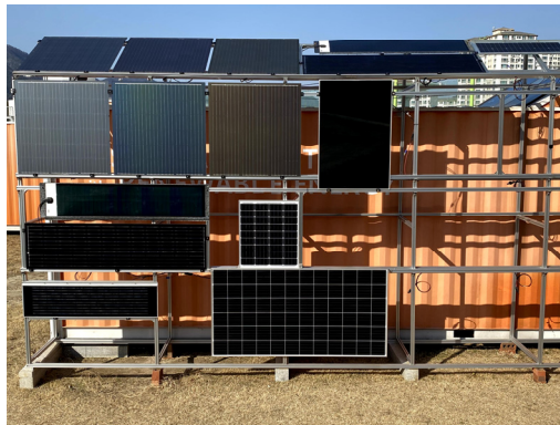
Fig. 2 View of the BIPV module performance test facility
