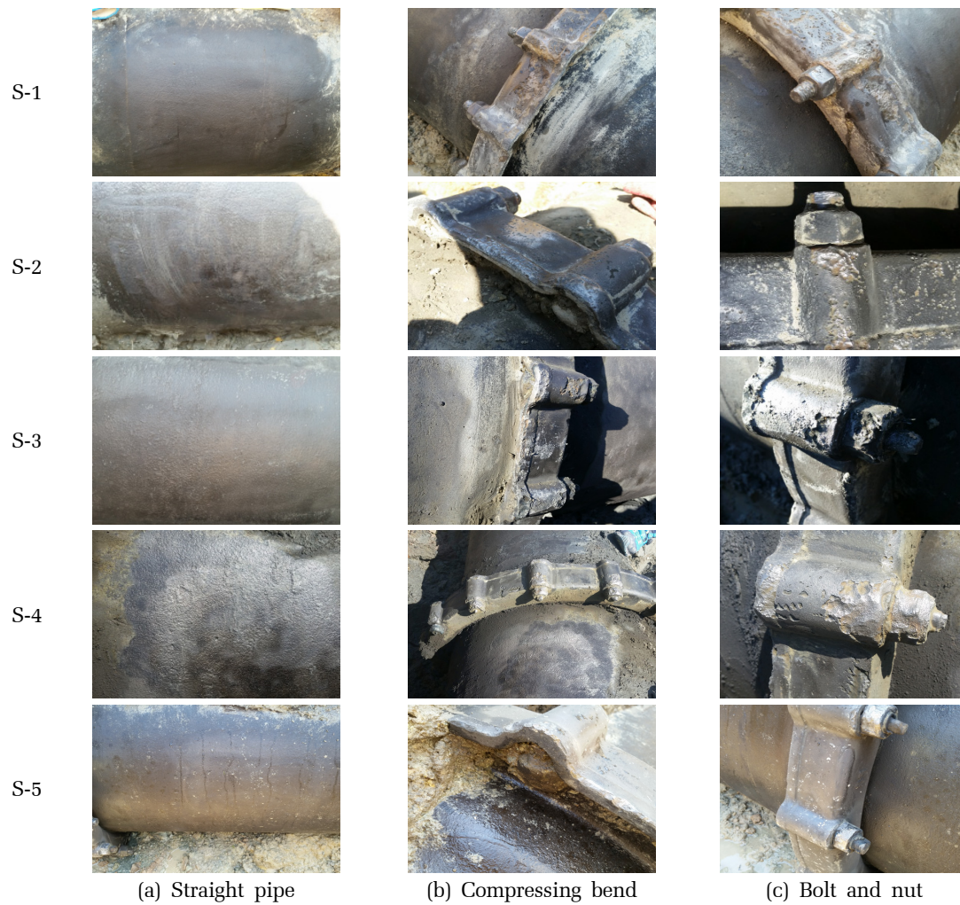
Fig. 3. Corrosion conditions of pipes, compressing bends, bolts and nuts at the sites(after abrasive brushing).
