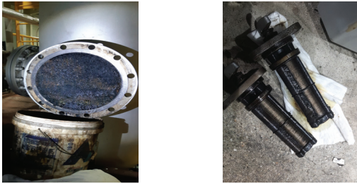
Fig. 2. Blockage by impurities (plumbing & filter).
