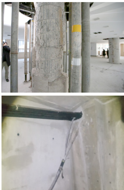
Fig. 1. Defects of Concrete Building and Bridge (Chosunilbo, 2019) (Seoul Metropolitan Government, 2017)
