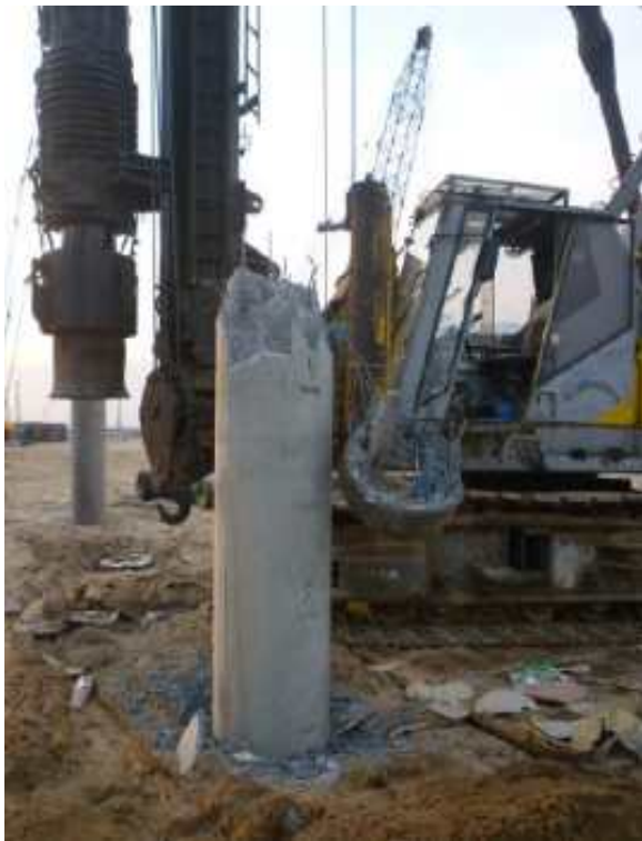
Fig. 5. Damaged pile head due to excessive hammer striking
