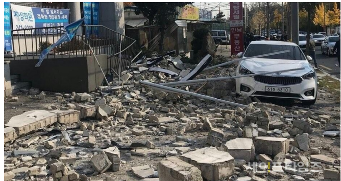
Fig. 8. Damage from the Pohang earthquake
