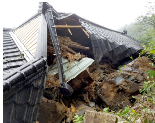
Fig. 6. Damage from the Gyeongju earthquake
