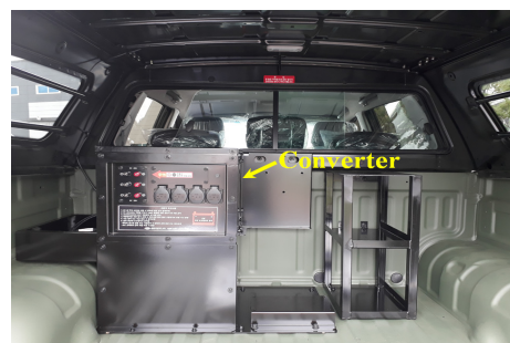
Fig. 2. Picture of previous power supply system
