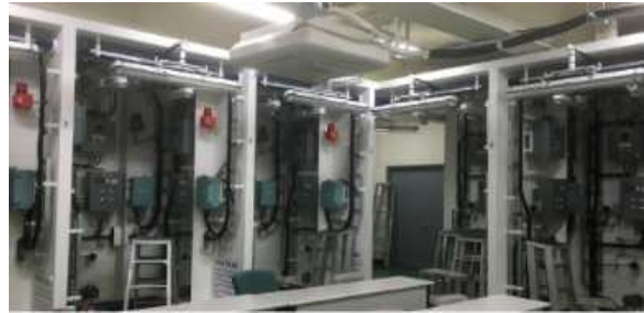
A Laboratory Booth for training of Production of Electrical Systems
