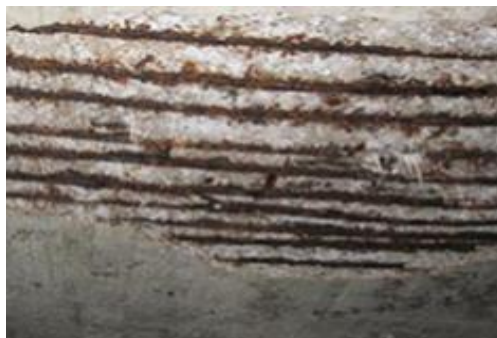
Figure 3. Concrete aging and rebar corrosion
