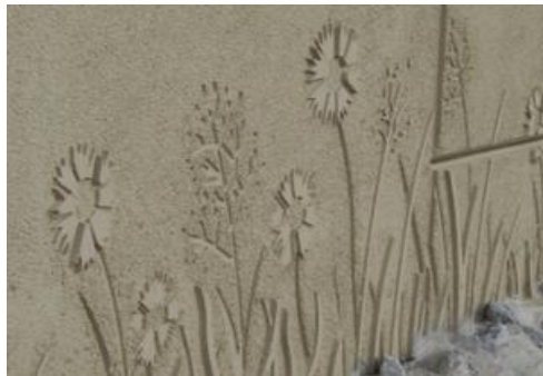
Figure 2. U.S. Case of Untreated Concrete Wall (Highway 161, USA)
