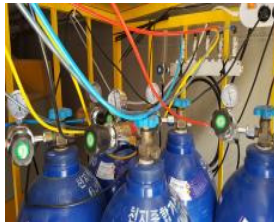
(b) CO 2 Tank
