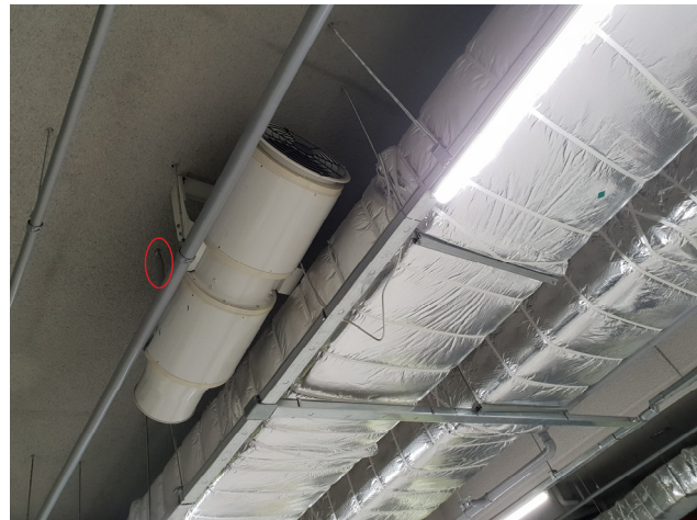
Fig. 2. Sprinkler head discharge obstruction
