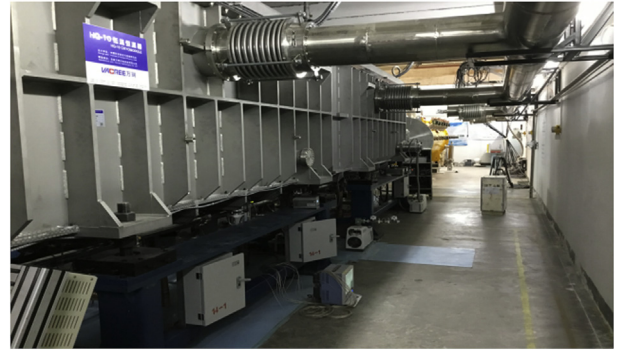
Fig. 12. Picture of the cryomodules with the HWR cavities installed in tunnel.
