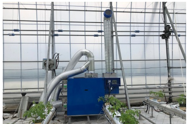
Fig. 2. Counter-flow Ventilator in greenhouse.
