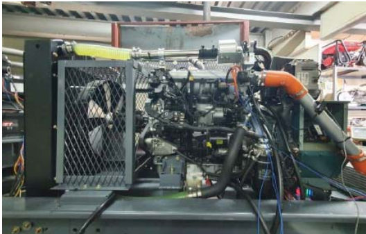
Fig. 1. Cooling fan control system installed in the engine generator
