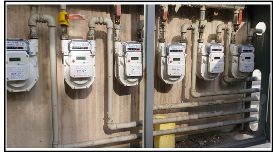
Fig. 8. Installed smart gas meter.
