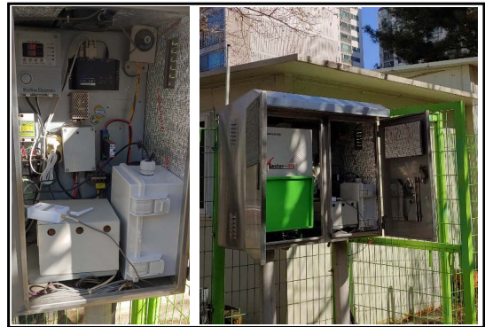
Fig. 9. Installed gateway for LoRa network.
