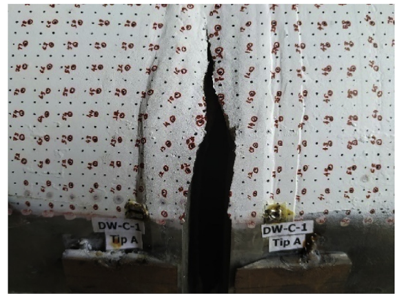
Fig. 6. Close-up view of crack location.
