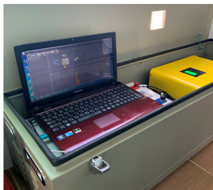
(a) Software operation picture in BESS
