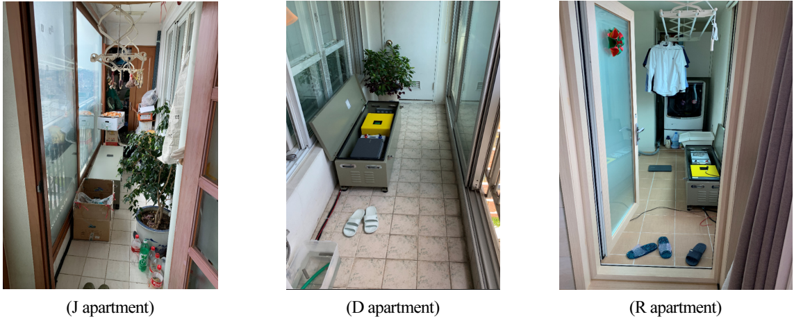
Fig. 5 Pictures of BESS installed on the balcony
