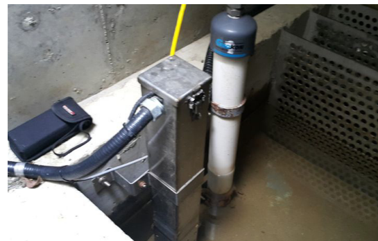
(b) Float level meter installed at the rear of V-notch
