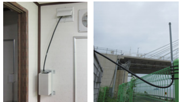
(a) LoRa gateway body in room (b) LoRa gateway antenna in outdoor
