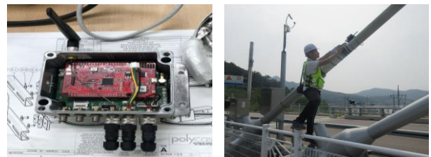
Fig. 3 DAQ board and installation
