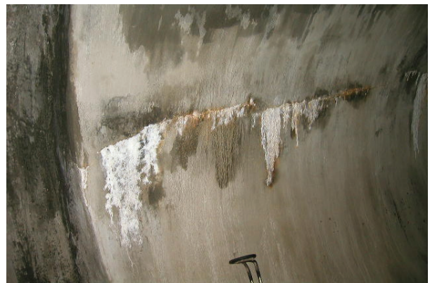
Photo. 1 Leakage in the Connection area of Concrete Structure
