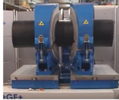
Figure 4. Pipe alignment in the chassis [6].
