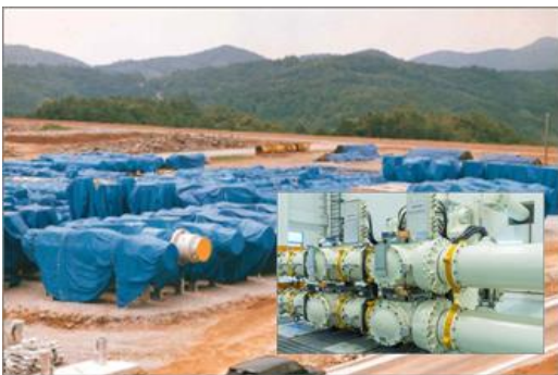
[Figure 5] Electric Breaker in outdoor storage
