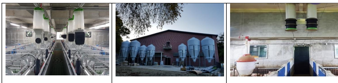
Figure 6. Smart ventilation system, Automatic supply system
