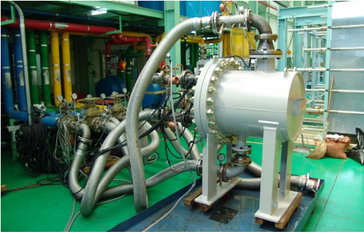
Fig. 6. Water-Water thermal performance test.
