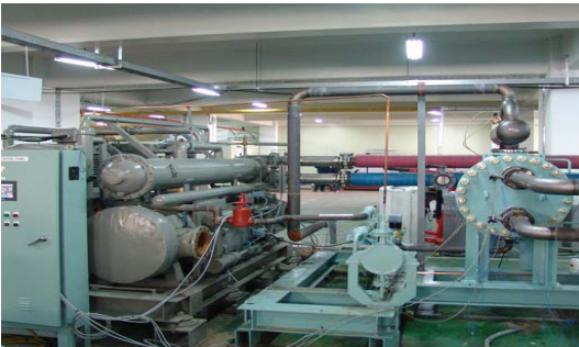
Fig. 11. 400 kW flooded chiller system.
