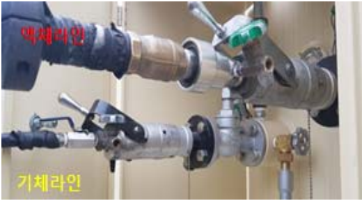
Fig. 6. LPG Supply system of Small LPG Storage with Bulk lorry.
