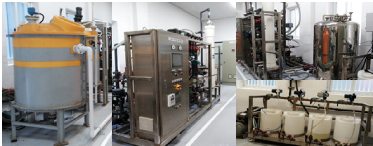
(a) Feed water Tank (b) Control Panel (c) Module skid(up) (d) Chemical tank(down)
