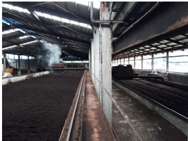
Mechanical-stirred composting facility
