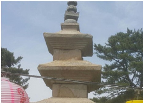
(a) Earthquake damage status of three story stone pagoda of Cheonryongsaji
