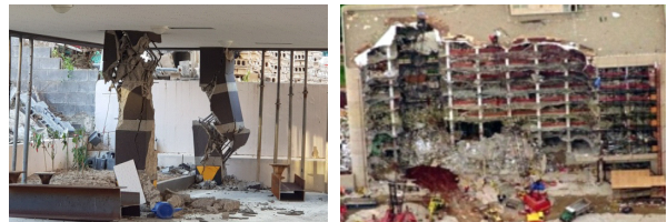
〈Fig. 1〉 Seismic and blast damage on building structures
