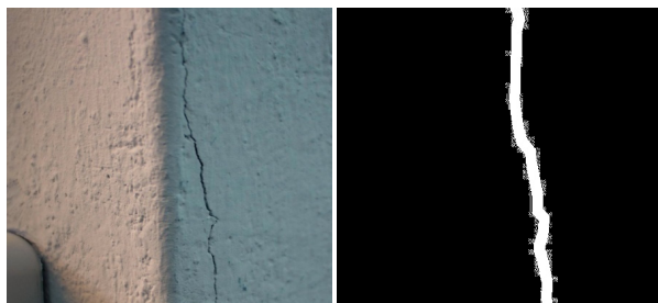
〈Fig. 8〉 Masking of cracks using crack images
