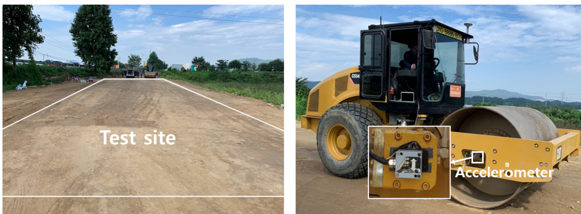
Fig. 5. Test site (left) and the accelerometer-equipped vibratory roller used in this study (right)
