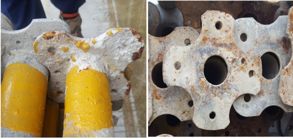
Fig. 3. Damage stamp (pipe support).
