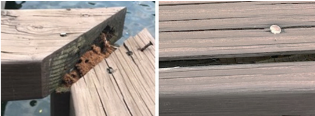
Fig. 3. The decayed parts of the cap rails.
