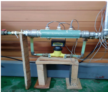
Fig. 3 Cold water chiller inlet and outlet temperature and flow rate measurement sensors
