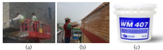
Fig. 10. Liquid type anti-absorption waterproof (a) Plaster (b) Spray coat (c) water repelling agents
