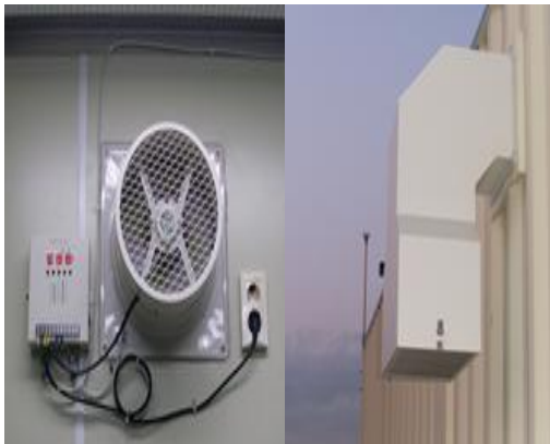
Fig. 9. 1Wireless Base Station Installation Site
