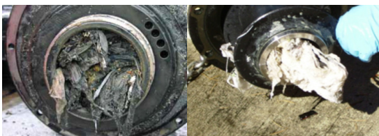
Fig. 1. Clogging problem of submerged pump
