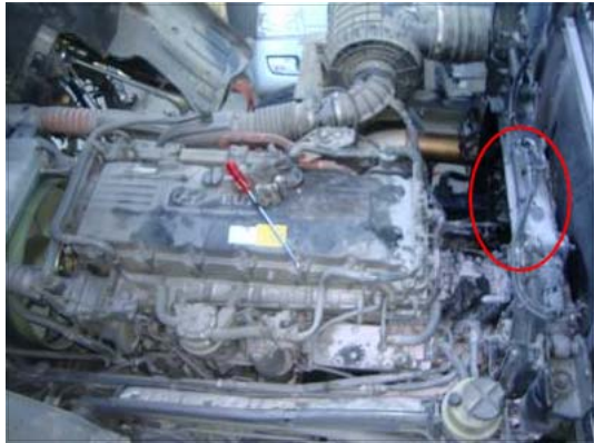
Fig. 5. Fire example of by wiring short of tilting motor part.
