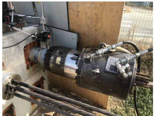
Fig. 9 Post Tension Jack Machine
