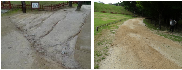
Figure 5. A Damage to the Viewing Road by Rainwater(Left) and Damage caused by Management Vehicles and Visitors(Right) Sunneung and Jeongneung in Seoul
