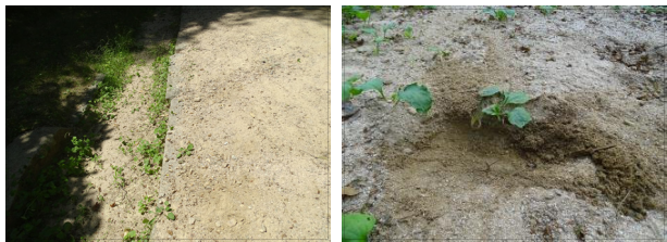
Figure 6. A Drainage Facilities buried due to Soil Loss(Left: Dongreung) and Surrounding Plants buried in the Lost Soil(Right: Seollung and Jeongneung in Seoul)
