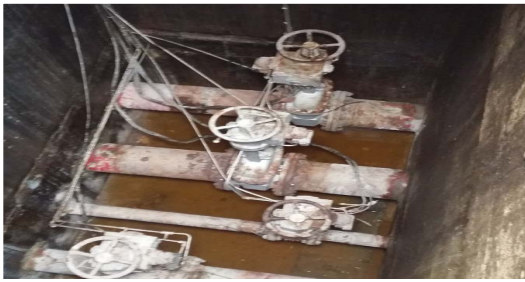
Fig. 4. A emergency shut-off valve.
