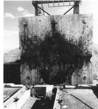
(b) Image of damaged concrete block
