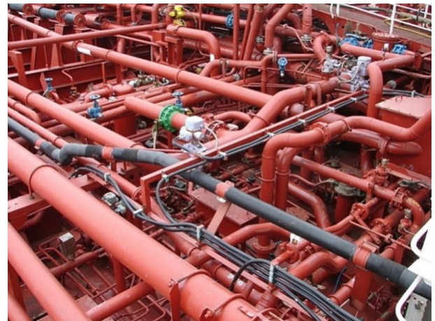
Fig. 2 Piping system of shipbuilding industry
