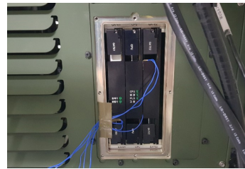
Fig. 9. Installation Enviroment of Gate 1,2
