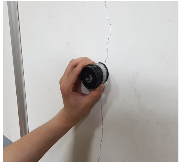
Fig. 8 Crack Width Measurement by Crack Gauge
