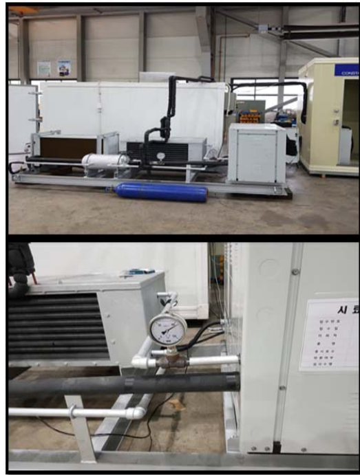
Fig. 11. High pressure piping for 120 bar.
