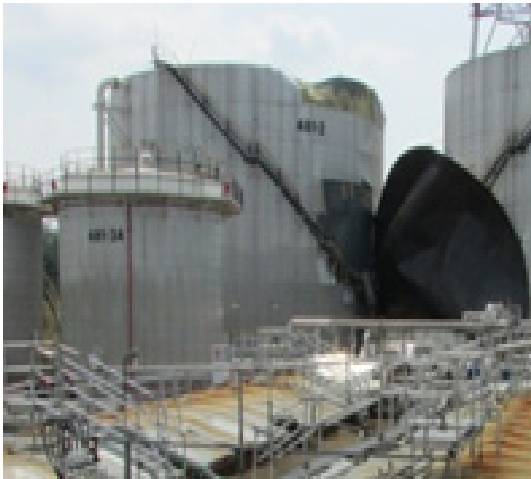
Figure 4. wastewater storage tank after explosion.
